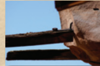
Close-up view of remaining wood beams of the Hanging Flume. Photo by Charles and Beth Smith
